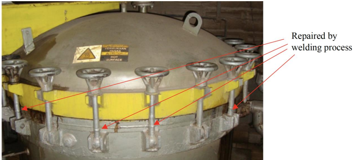
Fig. 1. Oil filter vessel indicating the numerous repaired bolts by welding process.
