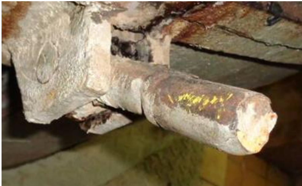
Fig. 3. Fractured bolt showing that ductile fracture was occurred.
