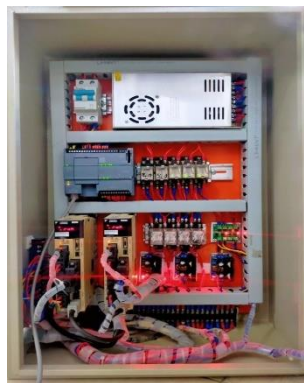
Fig. 21. Electrical Cabinet Control System
